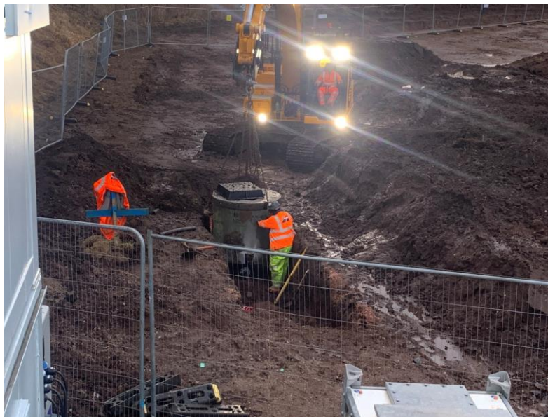
Rising Main Air Valve
